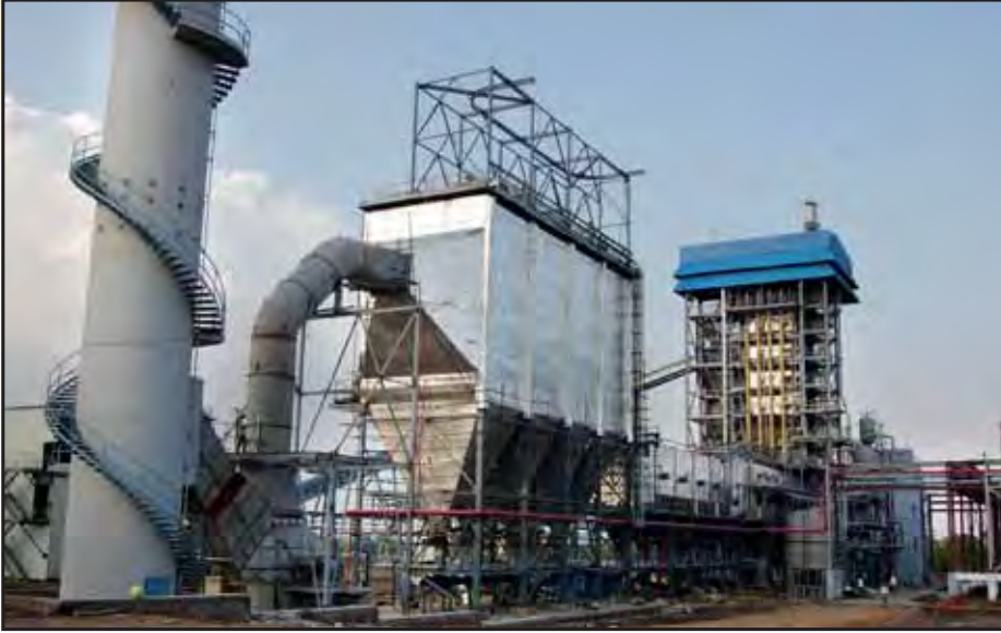
Incineration Boiler - Sameerwadi
