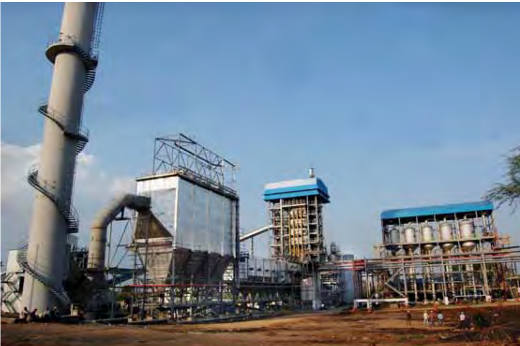
Incineration Boiler - Sameerwadi, Karnataka
